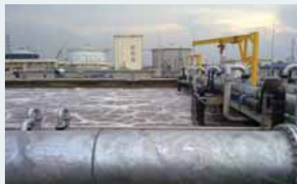
Wastewater treatment, Hanoi, Vietnam The wastewater treatment plant, Yen So Park, treats 50% of Hanoi's wastewater. More than 90 VSDs are installed, of which 12 450 kW VLT® AQUA Drives control the blowers.
